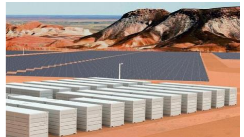
Source: Yadlamalka Energy is developing a 2 MW VRFB/ 6 MW solar project near Hawker, South Australia
